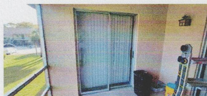
Unprotected glazed entry door
