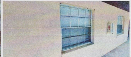
Unprotected glazed opening
