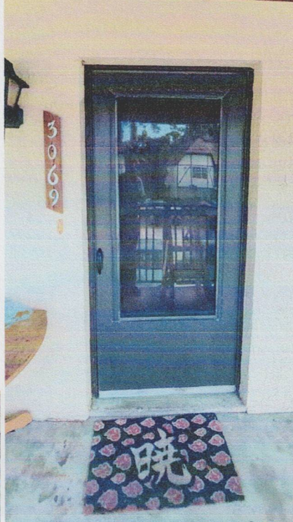
Unprotected non-glazed entry door
